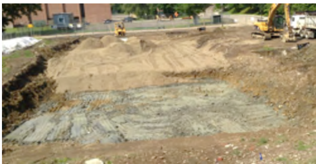
Figure 16. The clay layer extends from the Creek beneath the entire Ceramics Museum. Toward the right you can see it beneath the fill they put above.
