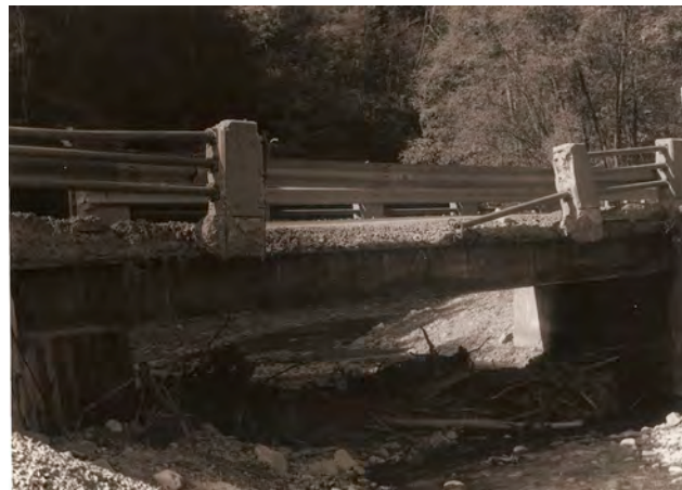
Figure 26. Old bridge, which served as a dam after debris lodged against it in 1984.
